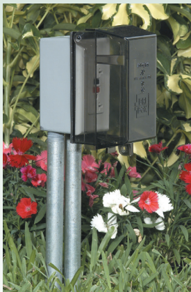
Why install boxes this way...
